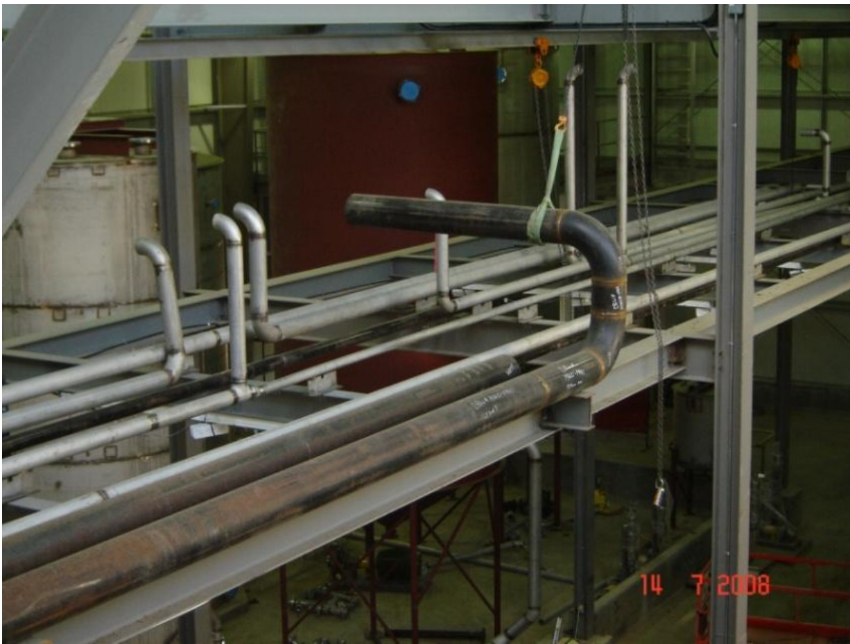
PIPING ON PIPE RACK
