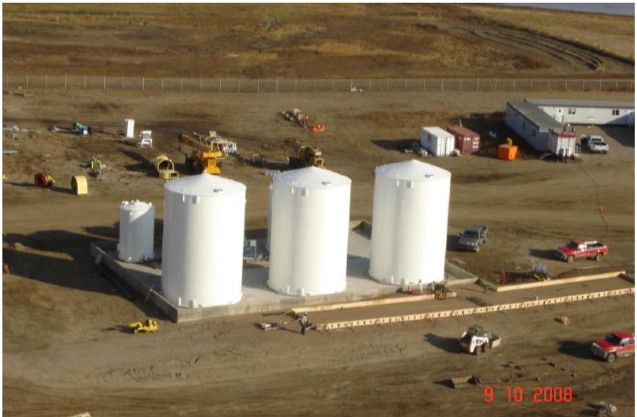
3 – 375,000 litre Ethanol Storage Tanks Totaling 1,125,000 litres
