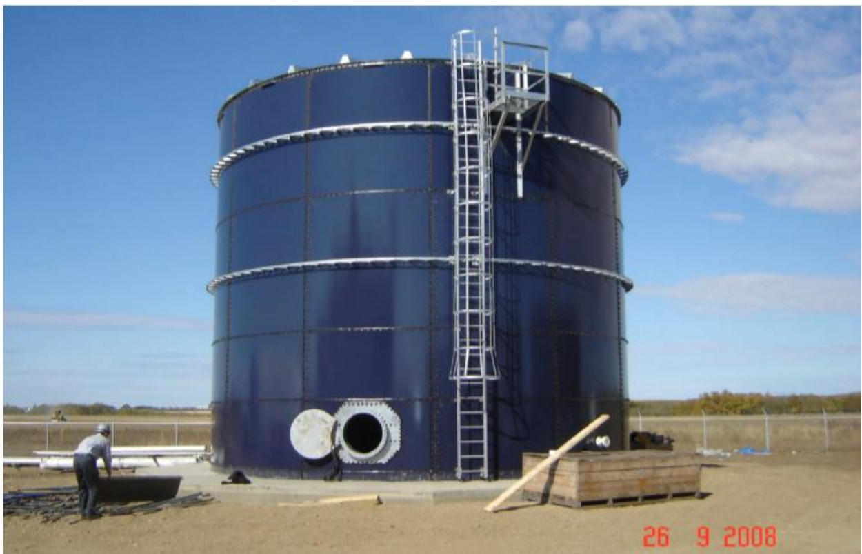
700,000 litre Fire Water Storage Tank
